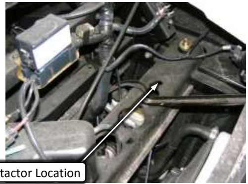
"Figure 11" Contactor Location
